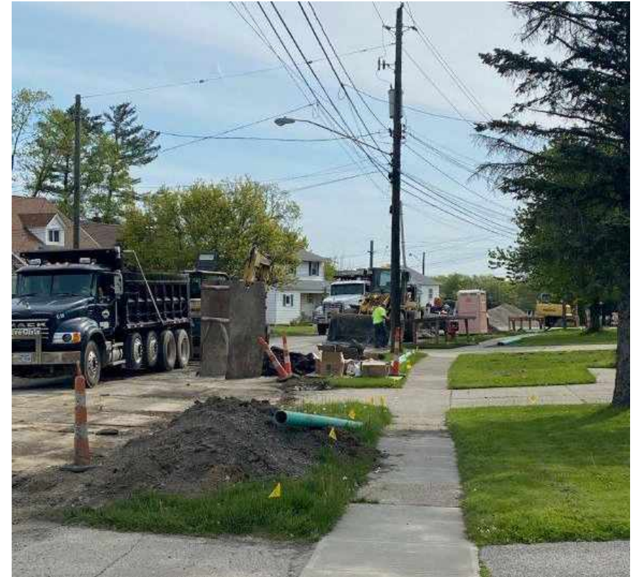
Such was the case here in this photo of the Chardon Avenue Rehabilitation Project.
